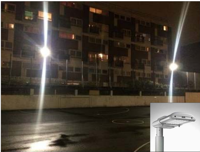
Photograph 1: Cree – LEDway Road Lantern at Margravine Estate, Field Road
